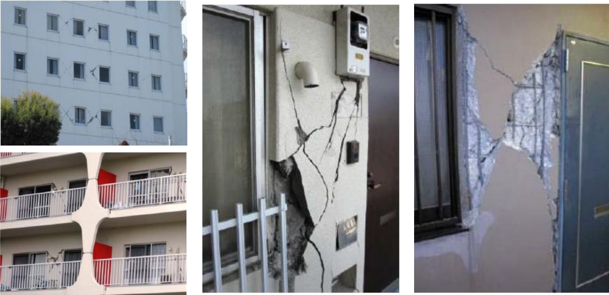
Figure 5-1 Damage of lightly RC walls after the 2011 Tohoku Earthquake [2]
