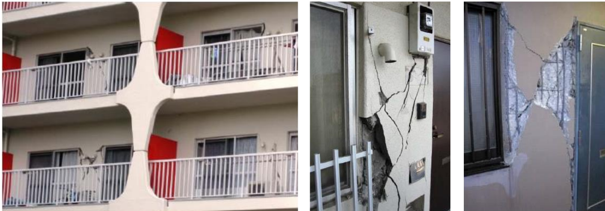
(a) Shear failure of lightly RC wall
