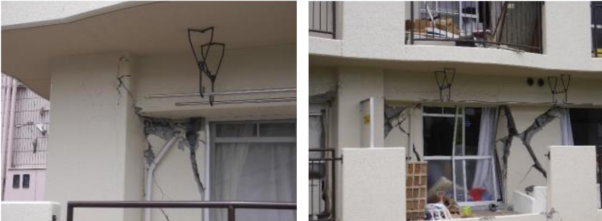
(b) Shear failure of wing wall
