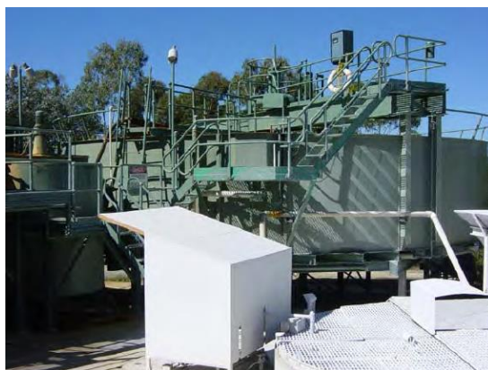
Fig. 1. 2 Low density sludge fixed plant [12].
