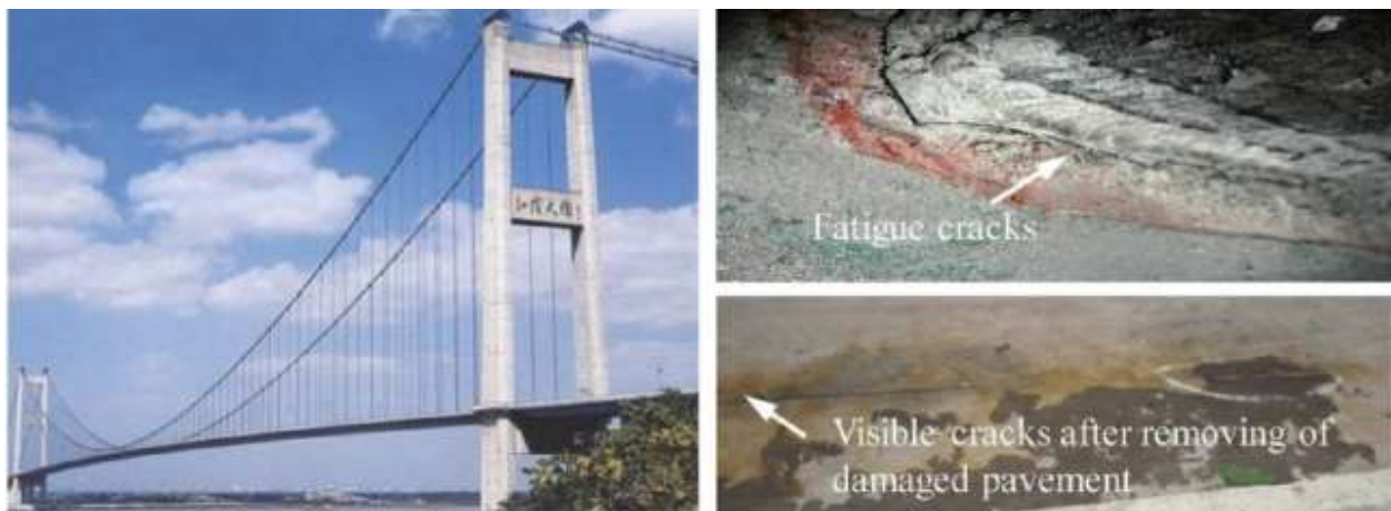
Figure 1.2 Fatigue cracks in Jiangyin Yangtze bridge [23].
