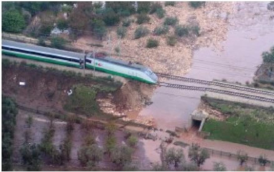
Figure 1.6 Breaching of the Acquaviva railway embankment, Southern Italy after 5 October 2005 flooding (taken from Polemio & Lollino, 2011)
