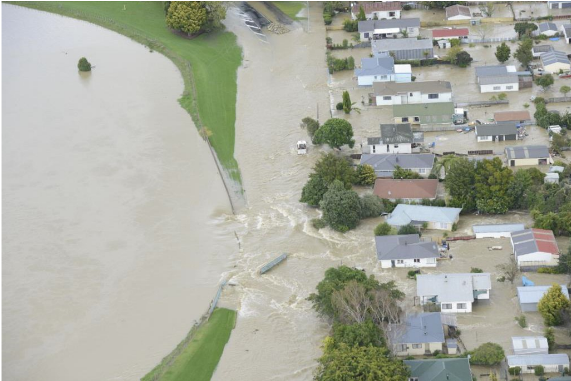
Figure 1.10 Breach of levee at Edgumbe, New Zealand, April 2017 ( Rangitaiki River Scheme Review- April 2017 Flood Event, 2017 )
