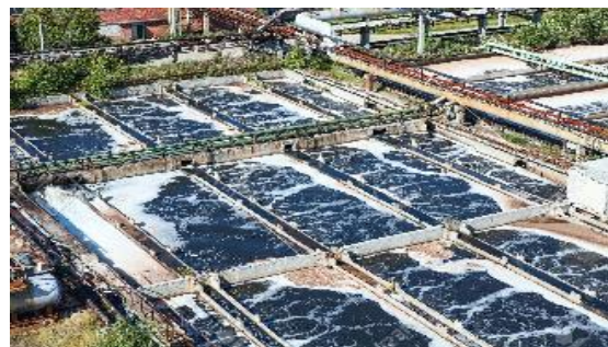
(b) Sewage treatment plant
