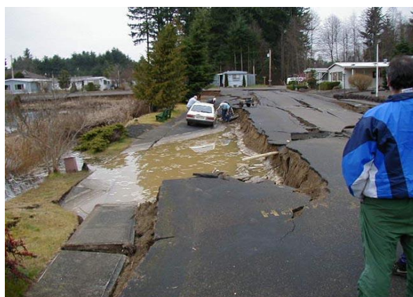
Fig. 1.6. Soil liquefaction and lateral spreading in Tumwater, WA after the 2001 Nisqually Earthquake (Courtesy of UW College of Engineering, USA)
