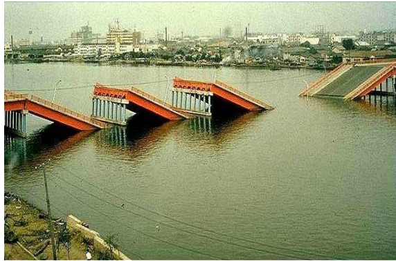
Fig. 1.4. The collapse of the bridge due to liquefaction induced lateral movement of the foundation during the 1964 Niigata Earthquake (Courtesy of the National Information Service for Earthquake Engineering, EERC, University of California, Berkeley, USA)
