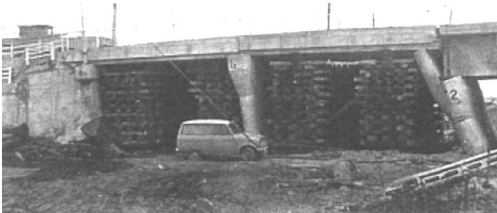
Fig. 1.7: Damages of Yachiyo Bridge during the 1964 Niigata Earthquake (Hamada et al., 1986).
