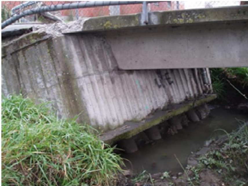
Fig. 1.10: Rotation of abutment of Porritt Park Footbridge (Waldin et al., 2012).
