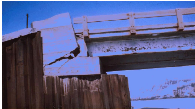
Fig. 1.3: Damage of abutment due to lateral spreading (USGS).
