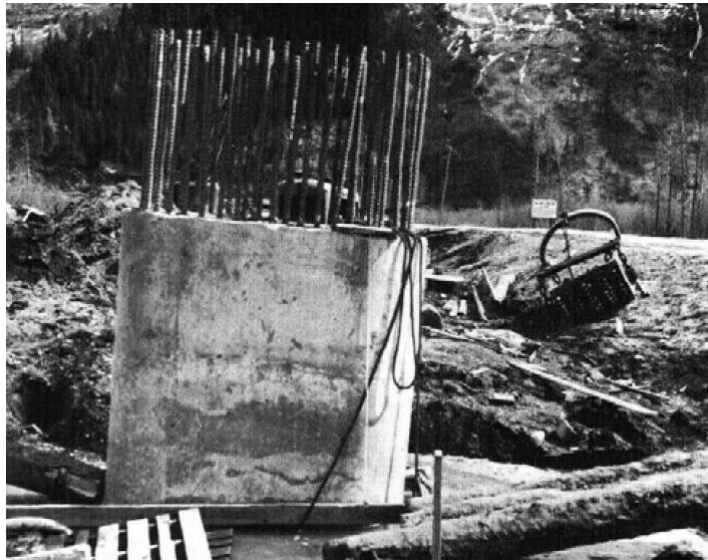
Fig. 1.4: Displacement of highway bridge pier supported on deeply driven steel piles at Snow River (McCulloch and Bonilla, 1970).
