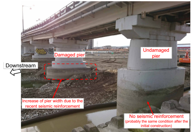
Fig. 44. Damaged pier during the restoration work (from downstream).
