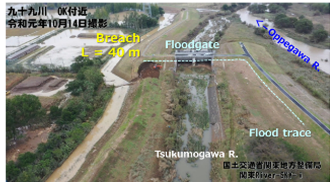
Fig. 6. Breach at 7.6 k on left levee of Opegawa River. The drone image was obtained from the database maintained by the Ministry of Land, Infrastructure, Transport and Tourism, Japan ( https://www.ktr.mlit.go.jp/bousai/index00000051.html ).
