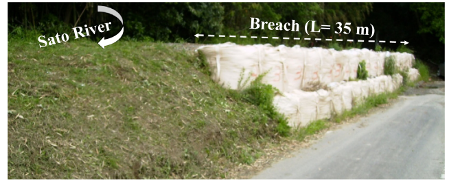
Fig. 33. Temporary restoration works of left levee of Sato River at Point B in Fig. 29.
