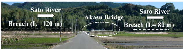
Fig. 30. Temporary restoration works of right levee of Sato River at Point C in Fig. 29 (near Akasu Bridge).
