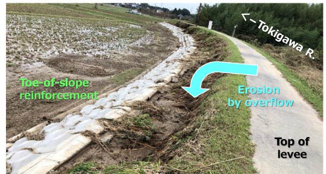
Fig. 11. Levee that survived erosion by overflow.
