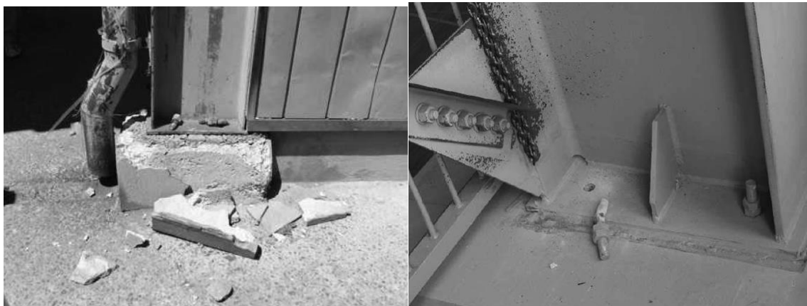
Photo 1-1 Anchor rods fracture in 2011 Tohoku earthquake [1-2]
