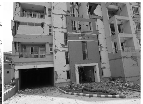
Photo 2 Out-of-plane failure of infill walls in the 2015 Nepal earthquake
