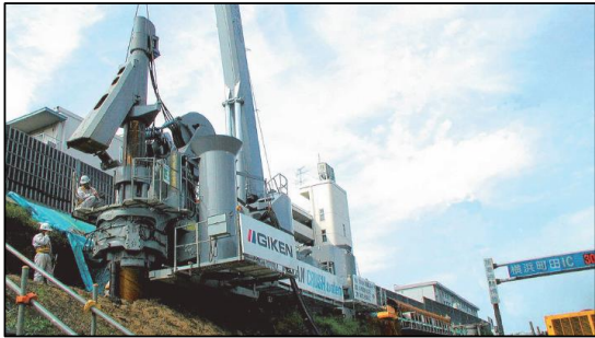
Construction of cantilever type embedded retaining wall in a narrow space adjacent to the highway with operation (Yokohama, Japan)
