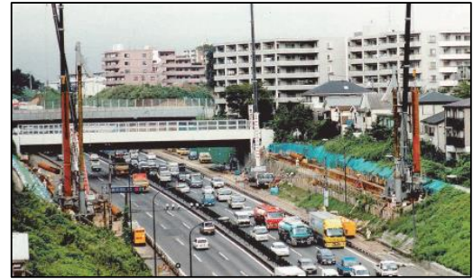
Pressing of steel tubular piles with 900 mm diameter in to mudstone (N-value of 166) to widen the existing highway (Yokohama, Japan)
