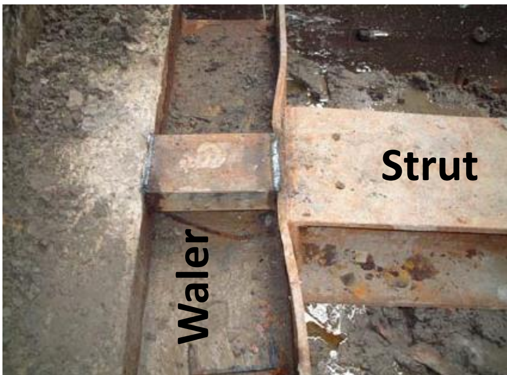
Figure 2.21 Strut and Waler buckling observed in Nicoll highway collapse incident
