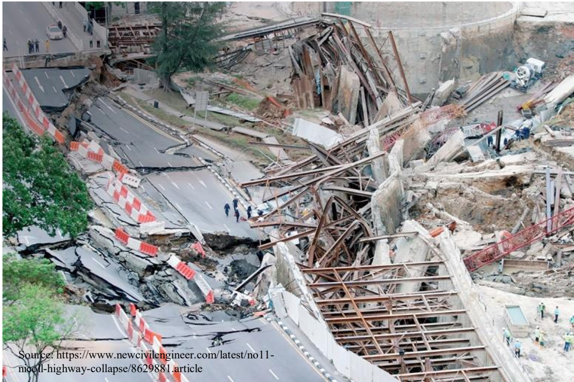
Figure 2.20 Nicoll highway collapse during the tunnel construction of an MRT line
