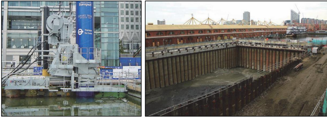
Construction of a subway station box in a canal (London, UK) Building of a cofferdam with high water cut-off performance using 1219 mm diameter tubular piles, Press-in application in to hard mudstone
