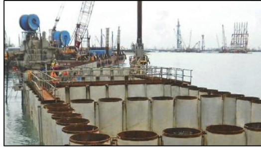
Cofferdam for revetment with 1200 mm diameter tubular piles installed in soft and hard marine clay (Singapore)
