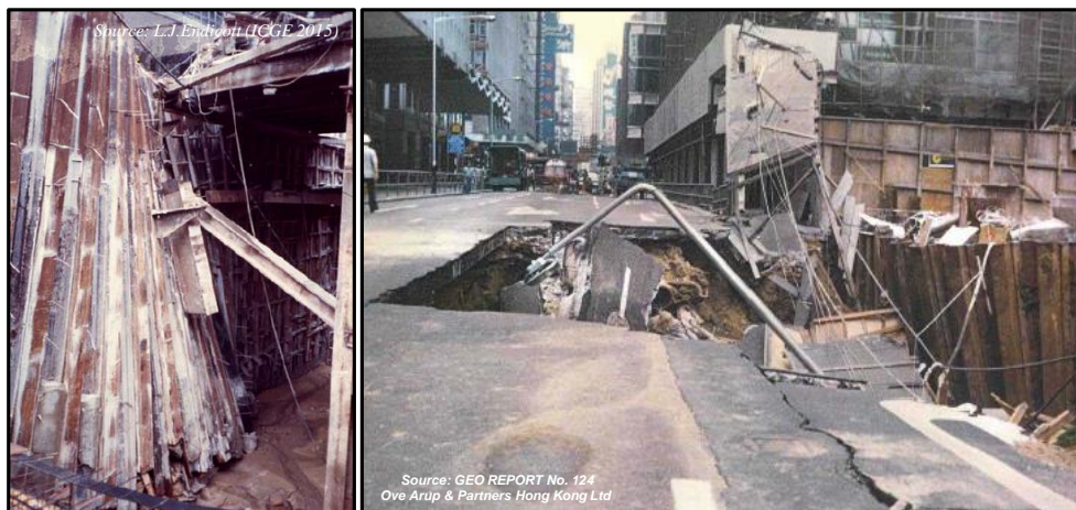
Figure 2.17 Sheet pile failure and Queen's road collapse during Edinburgh tower basement construction
