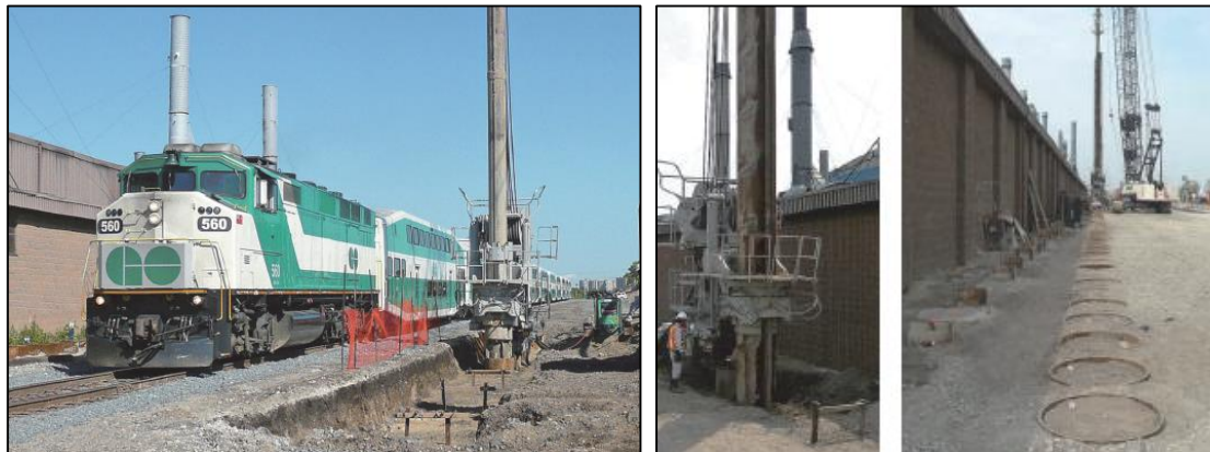
Steel tubular retaining walls for grade separation work related to a semi-underground railway in Toronto, Ontario, Canada. Press in tubular piles in to hard ground N-value greater than 160.
