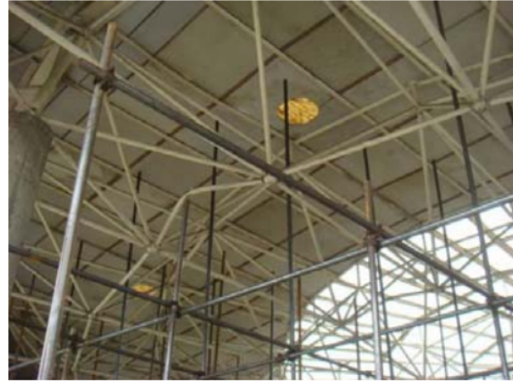
(b) Buckled roof members
