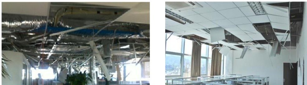
Photo.1 Damage of ceiling during Lushan earthquake in 2013
