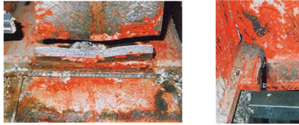
Fig.1.2 Fracture photos of beam-to-column connections in Kobe earthquake.[29]
