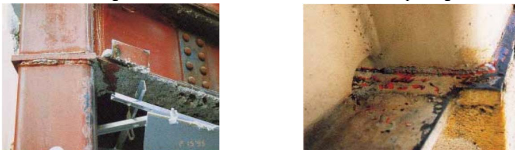
(a) Connection with horizontal oblique angle. (b) Connection with vertical oblique angle.
